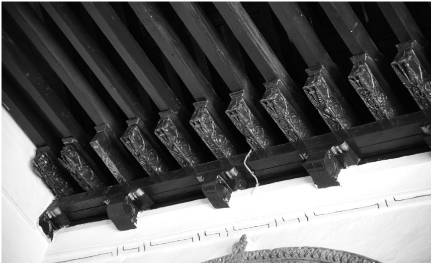
Figure 22. Detail of the support of the frame of the central nave (A. Almagro).
