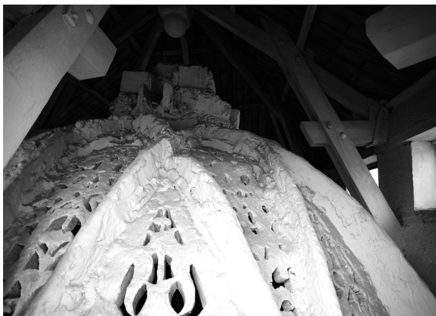
Figure 21. Detail of the extrados of the dome covering the maqşūra with the little top cupola (A. Almagro).
